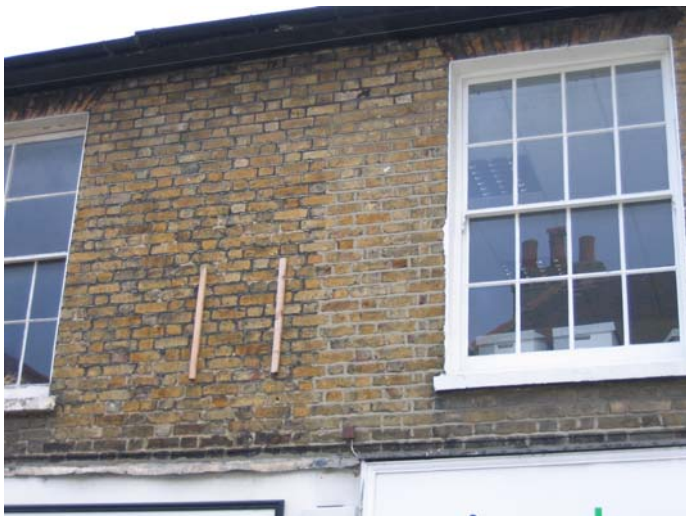
Fig 12 Nos 21-23 west Street. To the left, stock brickwork with tuck pointing. To the right, unnecessary repointing has had an adverse effect on the character of the brickwork.
