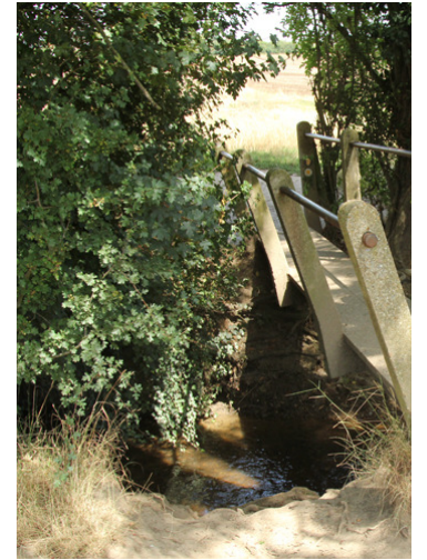
15 The Roach Valley Way crosses the River Roach via an informal pedestrian footbridge.
